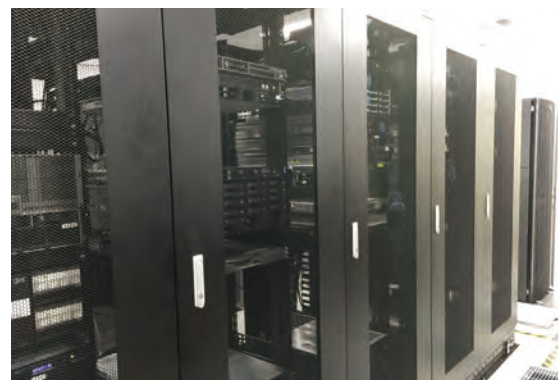
Information Center Server System. Our server stores data on approximately 6.5 million bioresources.
